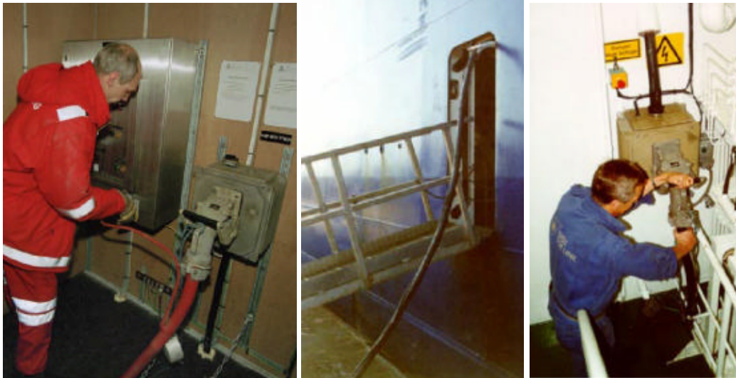
Figure 4 Connection practicalities (Photos: Port of Gothenburg)
